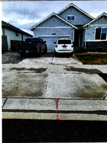
Rout-&-Seal All cracks
