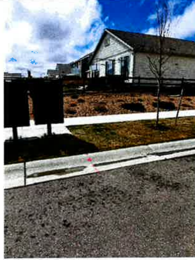
Make sure not holding H2O/Rout-&-Seal All cracks
