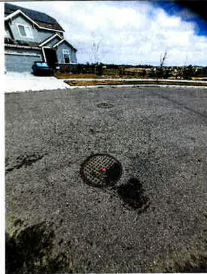
Wrong Manhole Lid Replace per Town of Mead Standard
