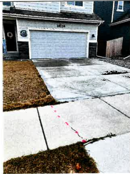
Rout-&-Seal All cracks
