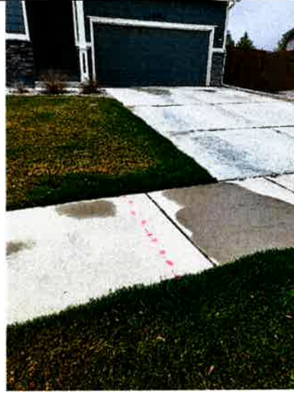
Rout-&-Seal All cracks
