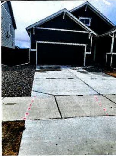
Rout-&-Seal All cracks
